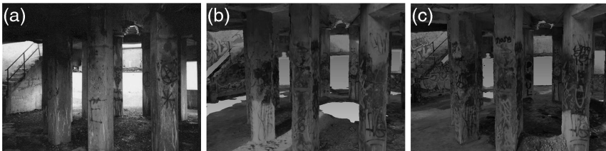
Figure 16.4 View of interior of radar building at Red Cliff, looking northwest; (a) May 1998; (b) February 10, 2018 (capture from Metashape model); (c) May 4, 2020 (capture from Metashape model).
